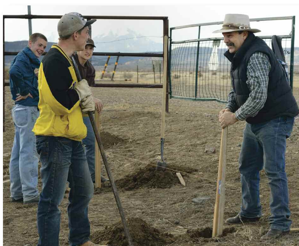
As Roy's family grew, he needed a bigger home. He and the boys are at work building a ranch in southern Colorado.
